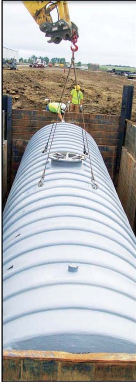
Above: After digging the pit with the slide rail system in place, workers lowered the 30,000-gallon storage tank through the clear-span opening.
