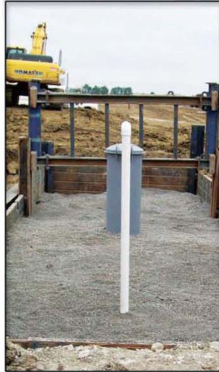
The top panels of the slide rail system supported the sides of the pit until all the work was done.
