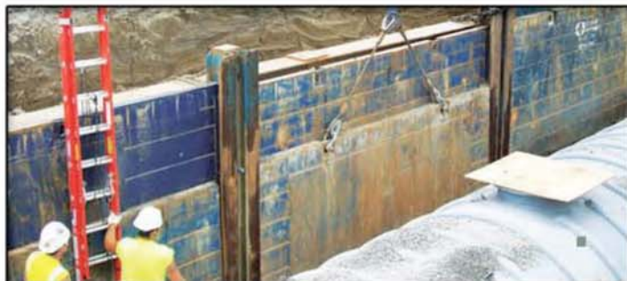
Above: Workers raised the slide rail panels gradually as they placed backfill in the pit.
